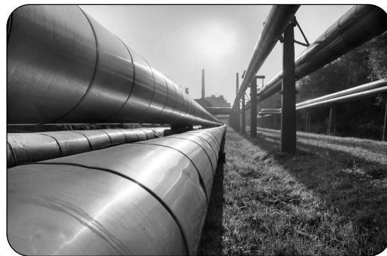
Pipelines are used to transport propane and natural gas to a processing facility.
