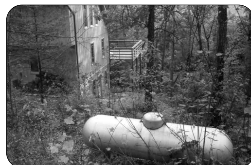
Propane is stored in a large tank. It is used to provide energy for heating, cooking, and drying clothes.
